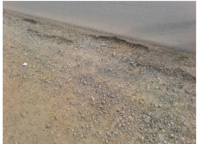
(a) Edge and Shoulder Damage
