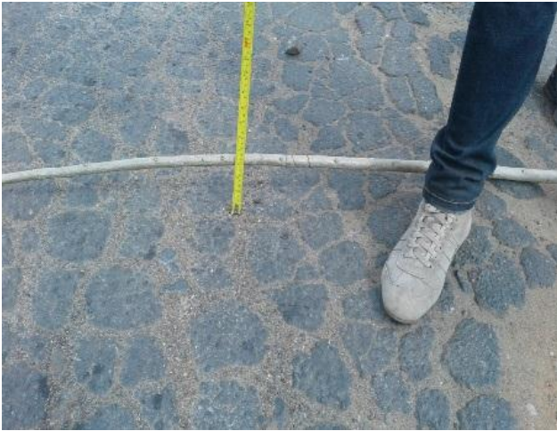
Plate 3. Rutting Btw. CH. 3+000 and CH. 3+500
