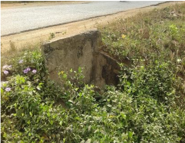
Plate 5. Culvert Inlet at CH. 4+500 Overgrown
