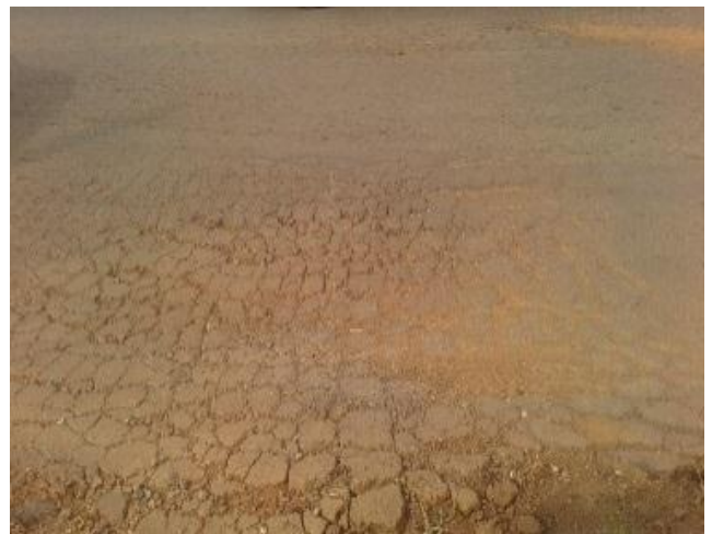
(c) Alligator Cracks
